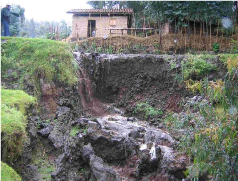
Figure 1: Severe erosion of volcanic soils in Rwanda. The steep pouroff is a headcut migrating up stream and across a road.
