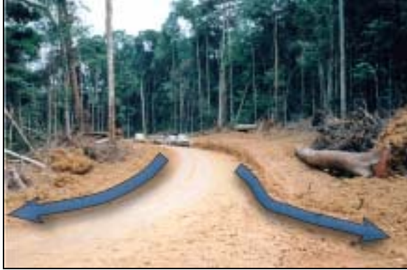
Photo 6. A primary logging road on the SBL concession in Gabon. The arrows trace evacuation ditches that divert water from the road surface and roadside ditches into the undisturbed forest.
