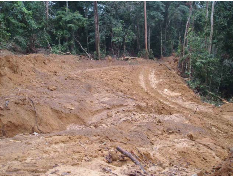
Photo 16- Road reconstruction (with major disturbance) due to poor road location.
