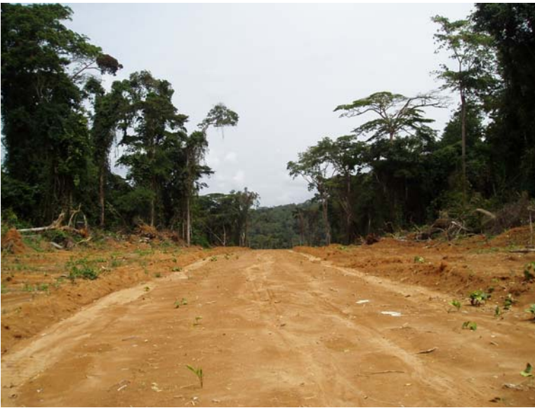
Photo 2- Excessive road and clearing width on a Local Road.
