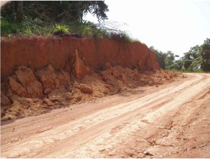
Photo 9- Unstable, slumping vertical cutbank.
