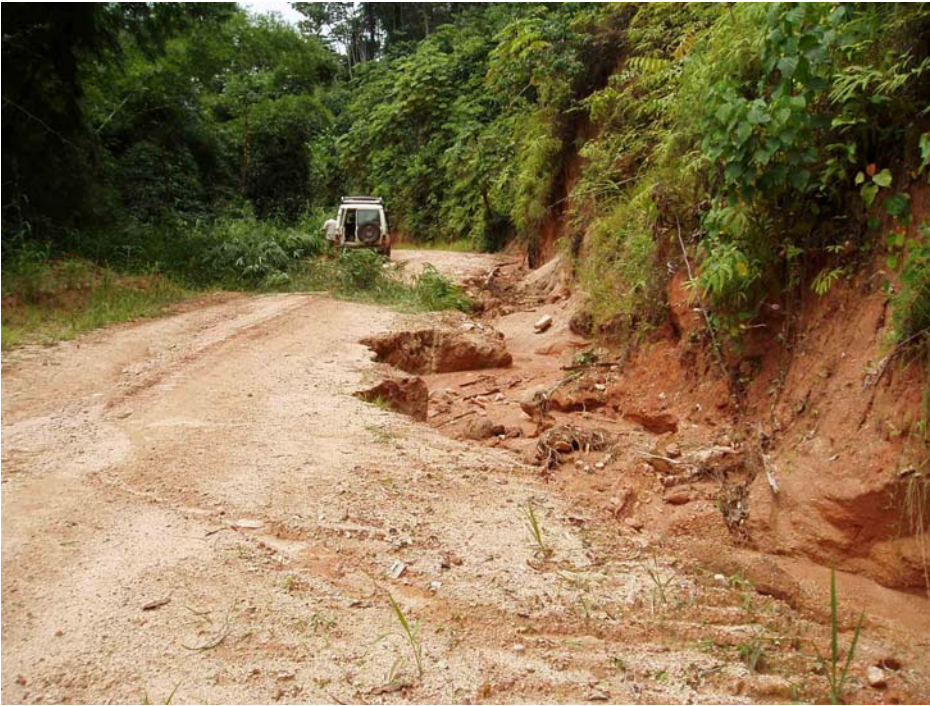
Photo 5- Ditch erosion caused by lack of surface drainage.
