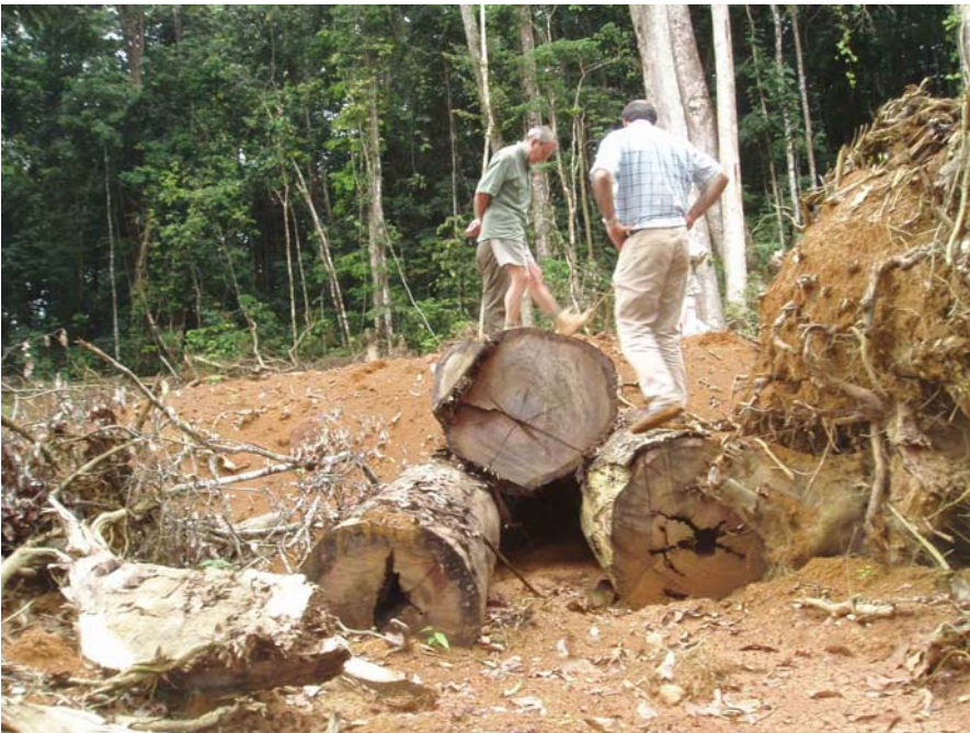
Photo 12- Commonly used log culverts-limited flow capacity, but inexpensive and appropriate for temporary roads.
