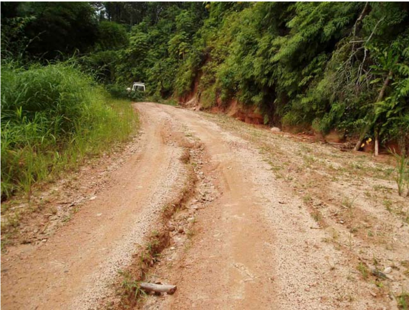
Photo 6. More surface erosion caused by concentrated flows and lack of surface cross-drainage.
