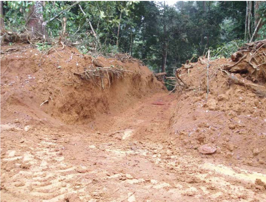
Photo 4- Deep leadoff ditches requires after excessive earthwork.
