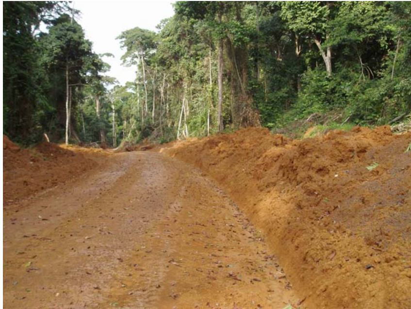
Photo 3- Excessive ground disturbance during new construction.
